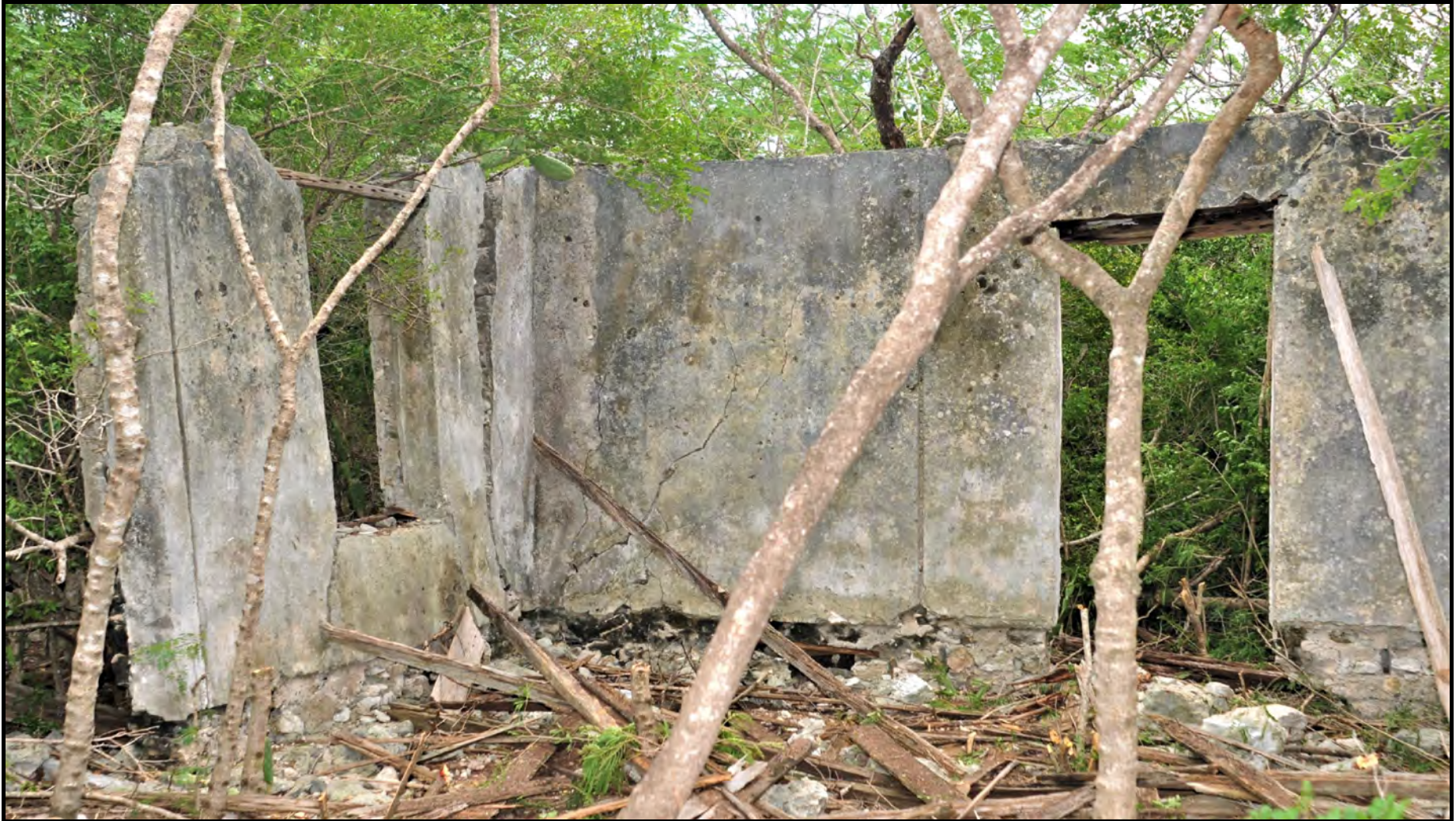
Plate 10. Structure 5. Interior view of southwest corner showing dangerous structural disassociation. Narrow vertical grooves in plaster represent otherwise lost timber internal partitions.
