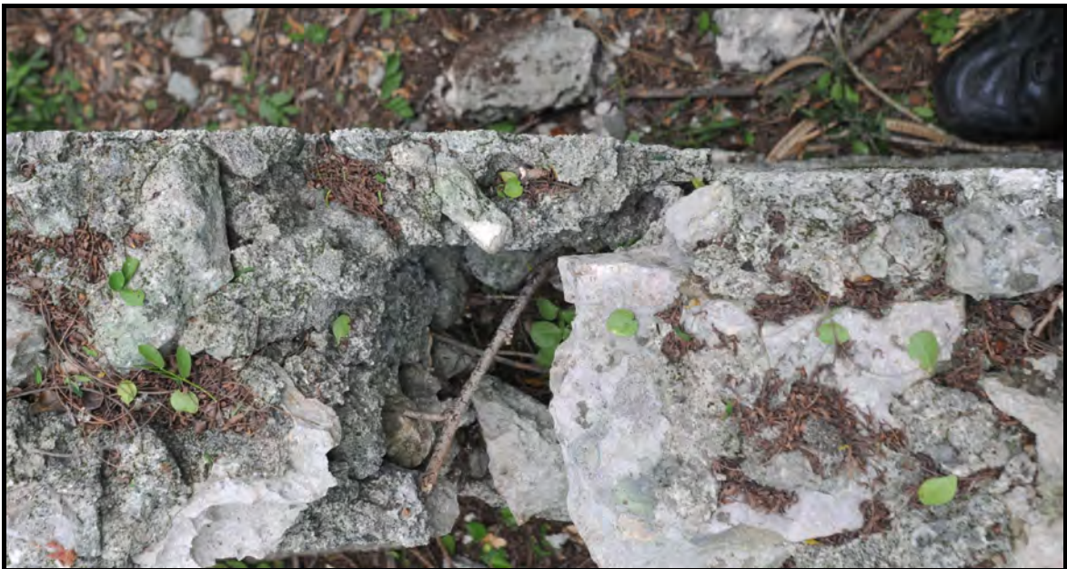
Plate 4b. Structure 2, south facade, plan view showing tabby and rectangular post hole.
