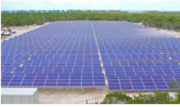
A new solar farm facility is currently underway on Castaway Cay and once complete will generate approximately 70 percent of the island's power.
