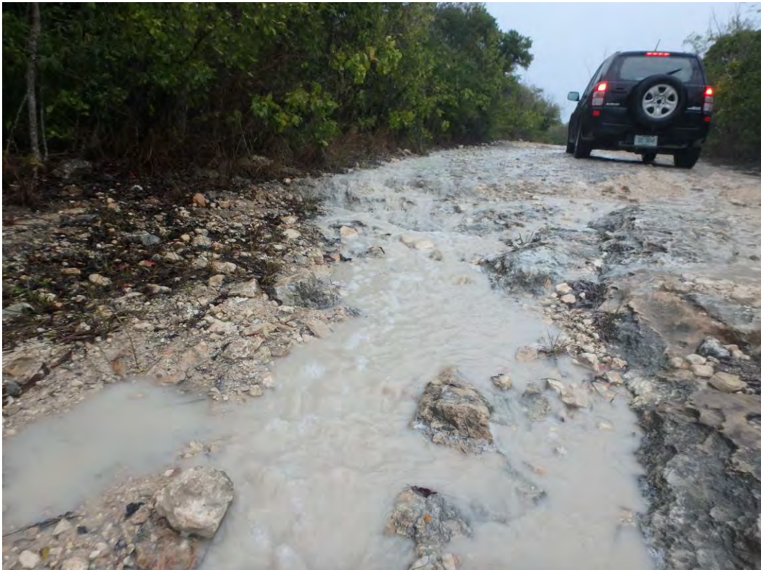
Photo 4-11. Deeply Rutted Road Through Center of the Site
