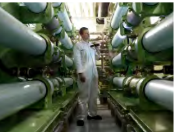
All Disney Cruise Line ships are equipped with Advanced Wastewater Purification Systems.
