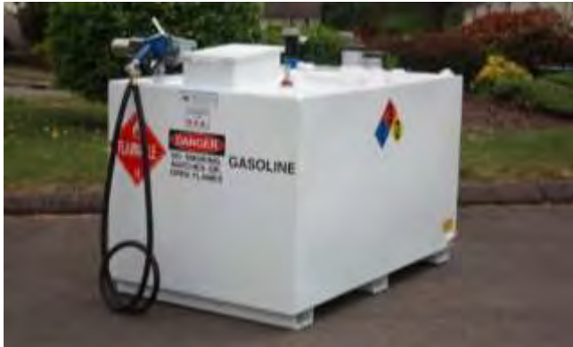
Photo 3: Typical 500-gallon double walled fuel tank. These tanks will be dispersed around the project to service any of the equipment working in each area. This could be on the trestle or in the upland areas.
